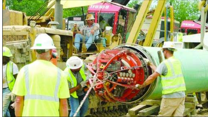
Workers use specialized equipment to make certain sections of the pipe are aligned.
